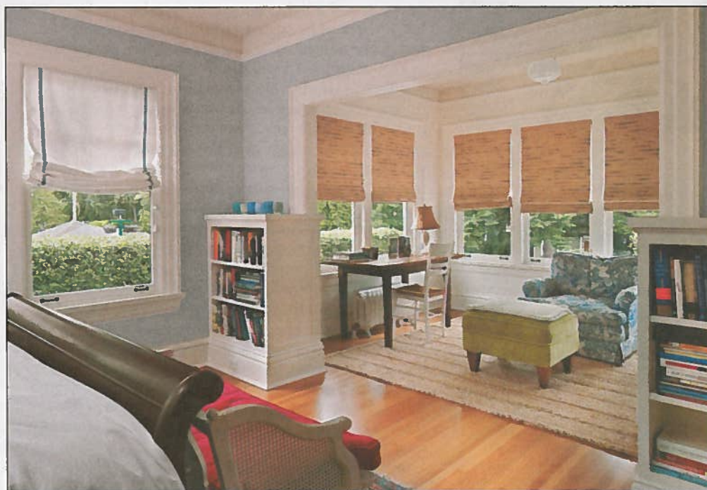
A dangerous old sun porch with a tar-paper floor and leaking windows was enclosed and rebuilt to create a sitting area in the master bedroom. Walls of windows and beadboard are reminiscent of the old space, but now it's useful and charming.
